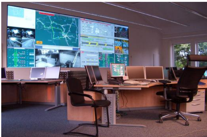
eyevis highways video wall installation, northern Bavaria
