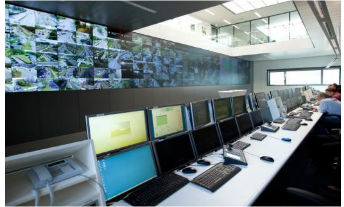
eyevis installation at Munich traffic management centre
