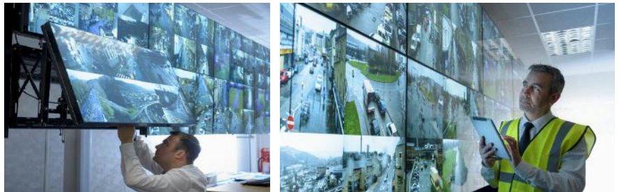
eyevis video wall installation at Calderdale Council CCTV Control Room
