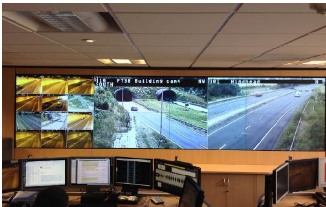
eyevis UK installation, Hindhead Tunnel operations centre
