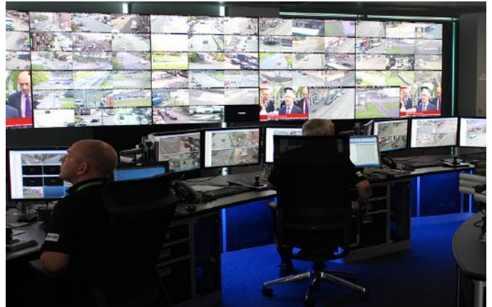
eyevis UK installation at Glasgow Council
